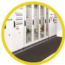
Electric Panel Floor Safety
